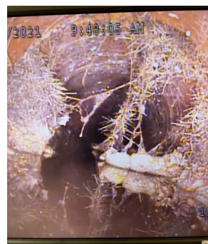
Roots & Grease in a lateral pipe
