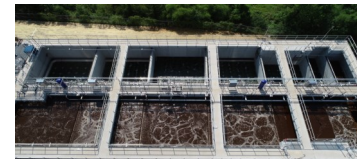
Activated Sludge Aeration Tank
