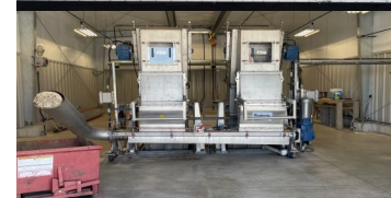
New Bar Screens
